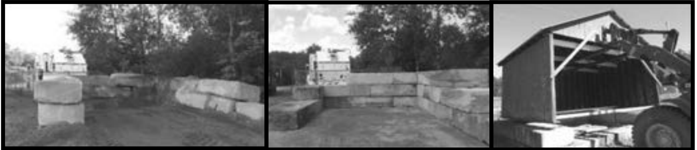
Left: The old bin before repurposing it for the new location of the community sand/salt shed.
