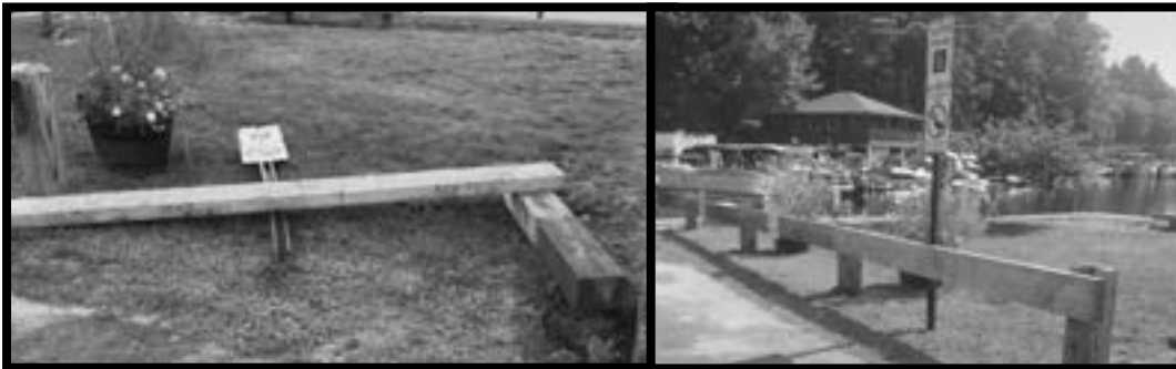
Left: Guardrail, that was previously repaired, after withstanding a Memorial Day weekend collision.
